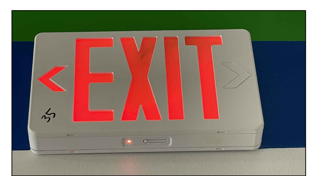
EXISTING EMERGENCY FIXTURE PHOTO (NOTE 3) NO SCALE
